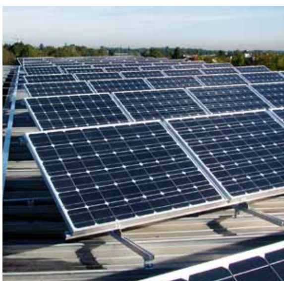
Roof-top plant Bergsionschule, Germany
