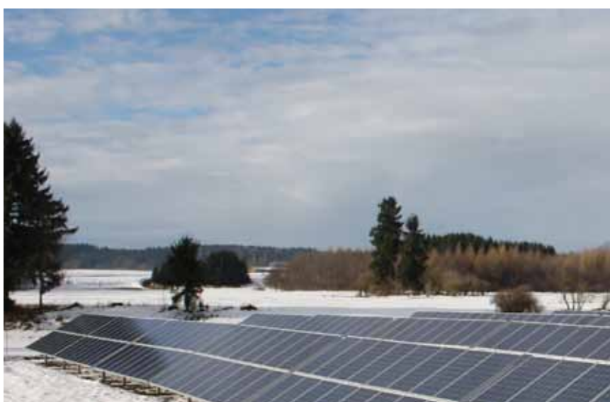
Photovoltaic plant Landsberg, Germany
